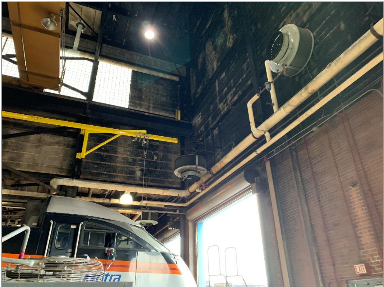
Figure 84 - 47th Street Shop Heaters – Steam Heat / Blowers
