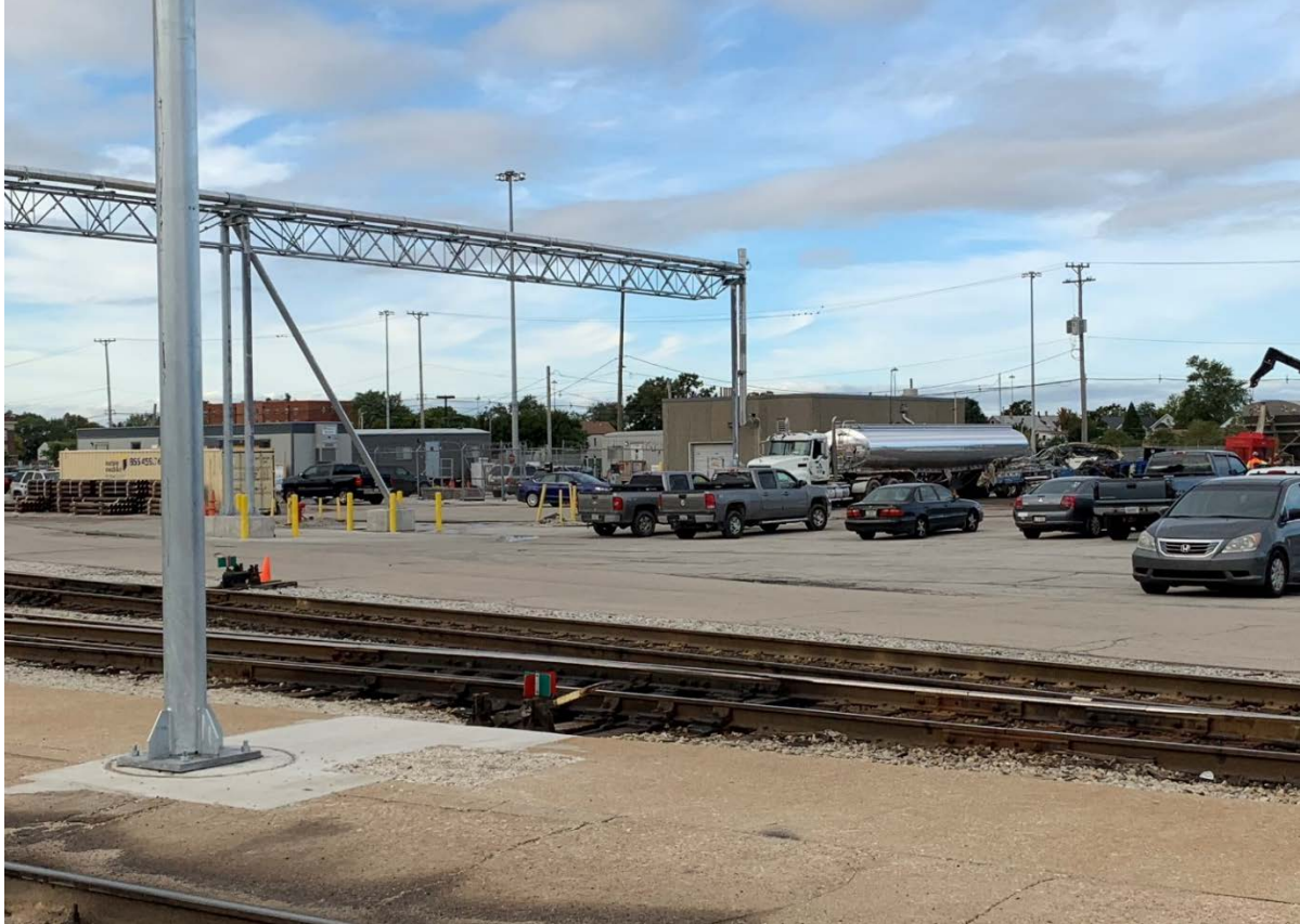
Figure 3 - Fuel Rack Supply Gantry and Pumping Station
