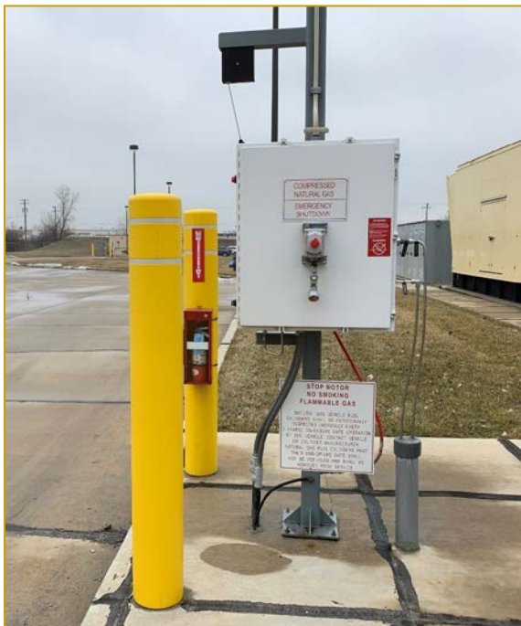
Figure 45 - Bus CNG Tank Evacuation System Connection
