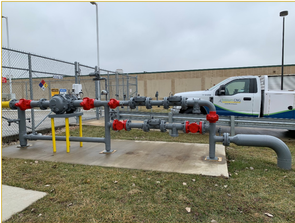
Figure 35 - Nicor Incoming 8" Line with Downstream Valves and Pressure Regulator
