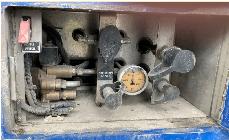
Figure 43 - Bus CNG Fill Manifold
