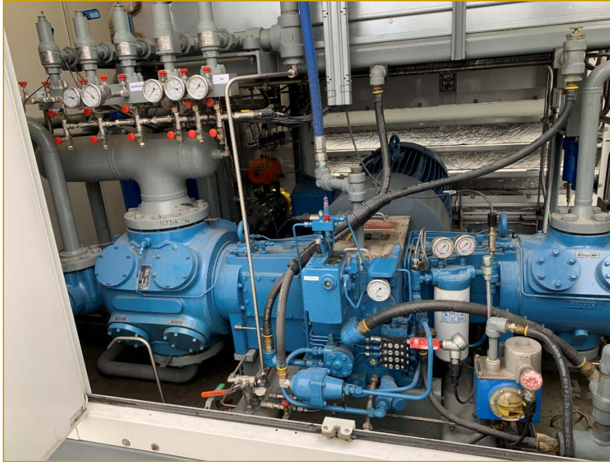
Figure 38 - Interior of Enclosure showing multi-stage pumps
