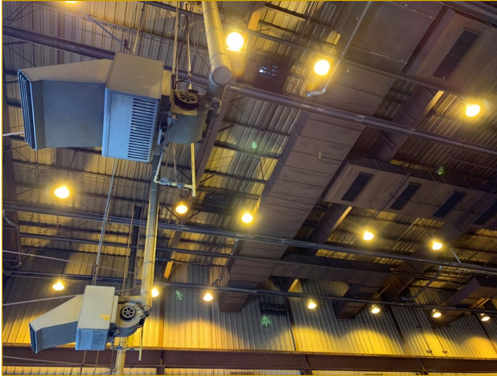
Figure 87 - Bay Door Heater Blowers
