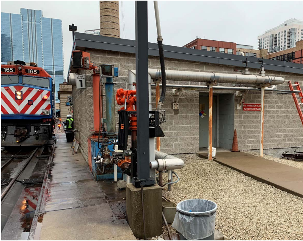
Figure 15 - Ogilvie Transportation Center Track 1 Fueling Racks
