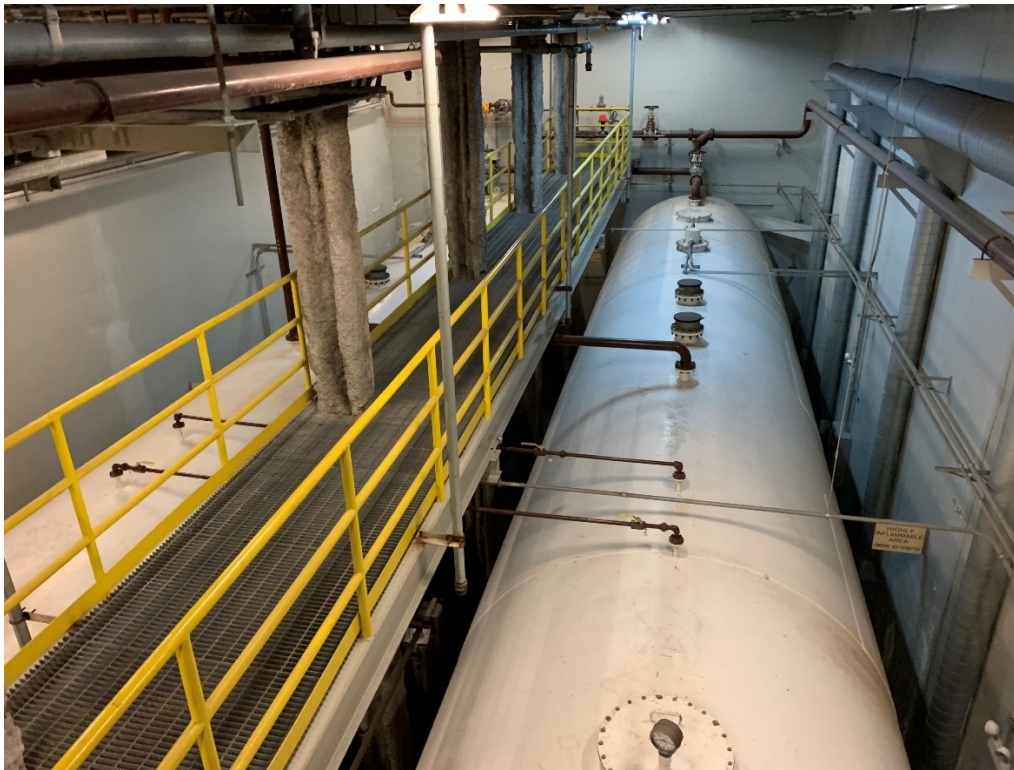
Figure 16 - Ogilvie Transportation Center Fuel Storage Tanks
