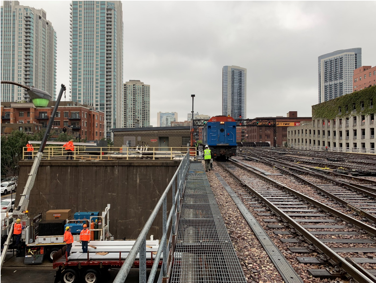
Figure 14 - Ogilvie Transportation Center Track 1 Fueling Facility
