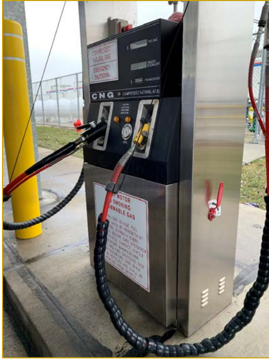
Figure 44 – Fueling Dispenser (2000 and 4000 psi capability)
