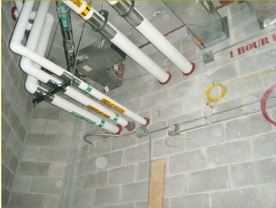
Figure 75 - Example of Sealed Penetrations
