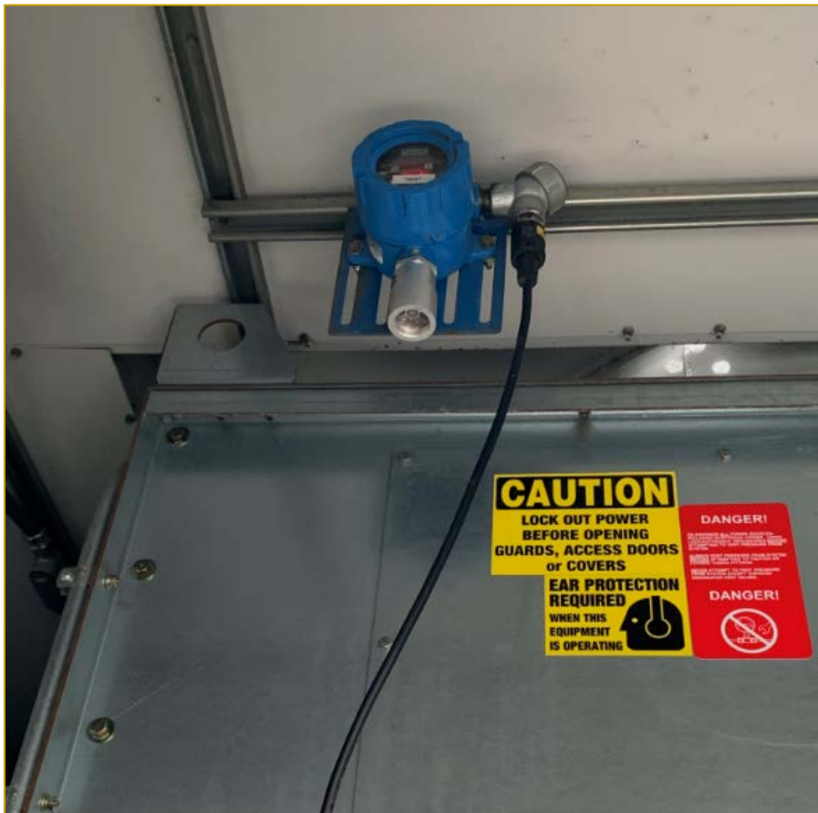
Figure 39 - Methane Detector inside of pump enclosure
