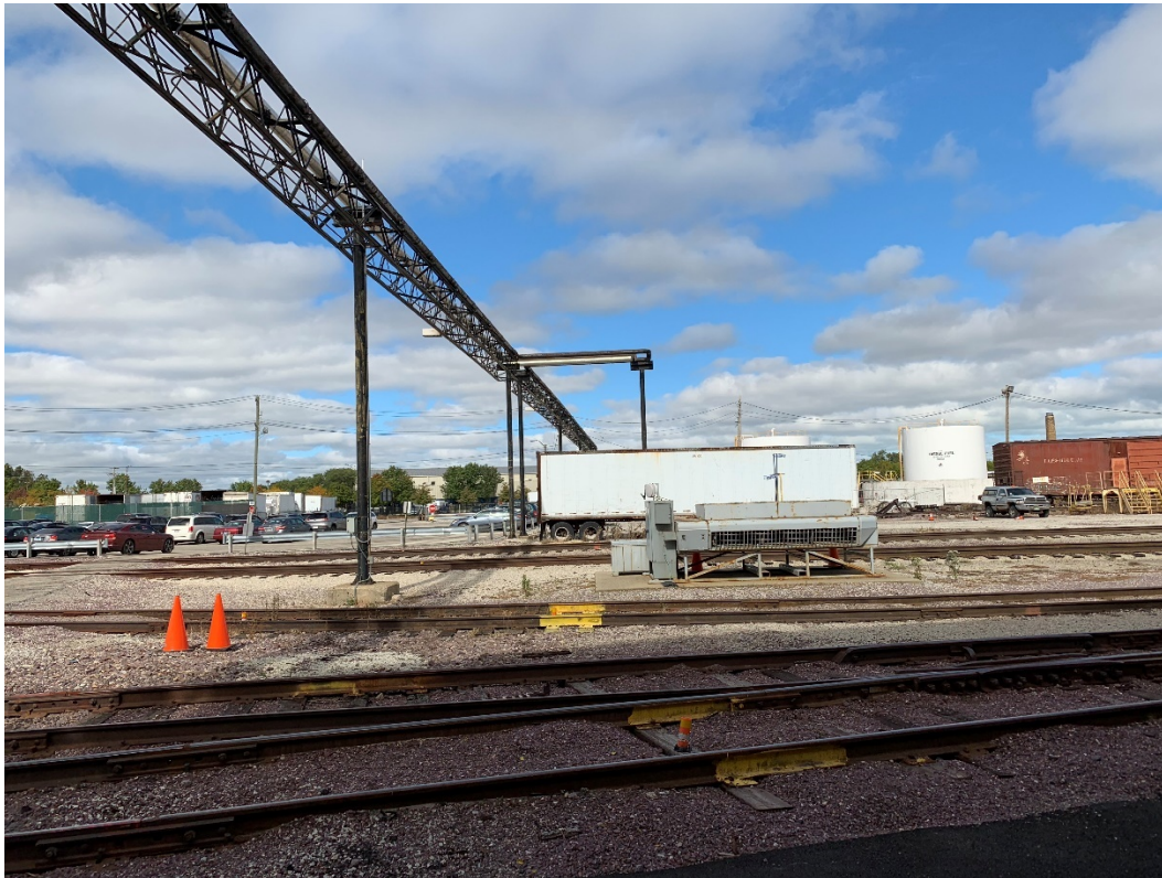
Figure 11 - M-19-A Fuel Pipeline Gantry
