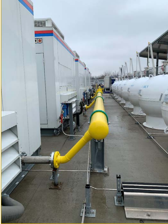
Figure 42 - Compressor Modules Feed (Yellow Pipe) and Output (Stainless Pipe) with Buffer Tanks
