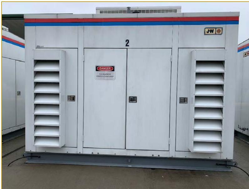
Figure 37 - Pre-Packaged Compressor Enclosure
