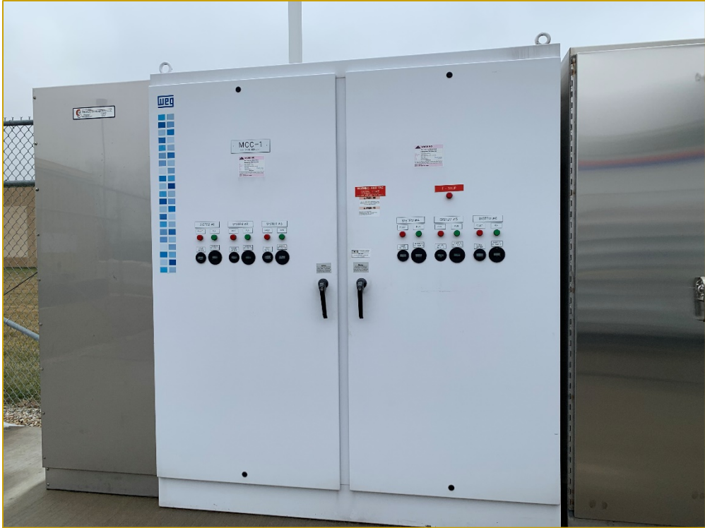
Figure 40 – MCC and Main PLC Cabinet
