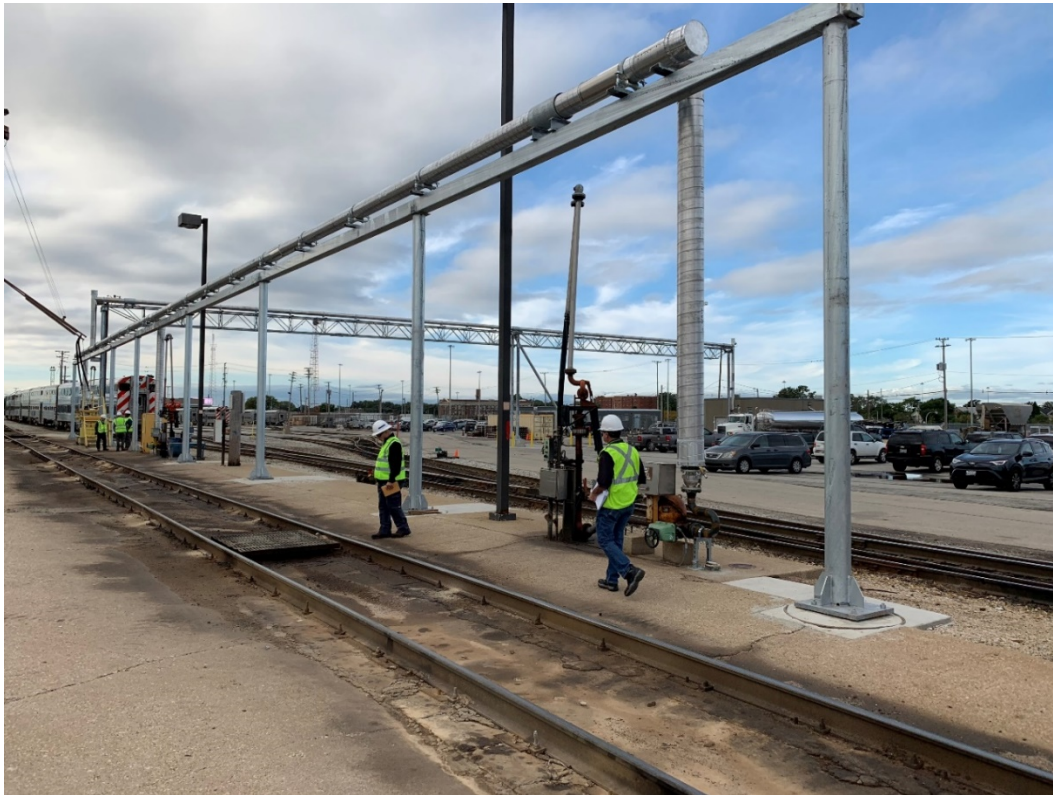
Figure 2 - 47th-49th-51st Street Yard Fuel Rack
