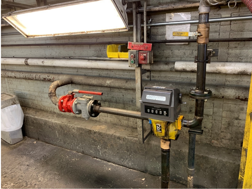
Figure 10 - M-19-A Interior Fuel Flow Meter (typical)
